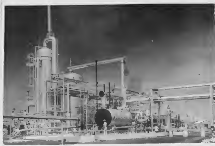
SULPHUR PLANT went on stream July 20 to make elemental sulphur from refinery fuel gases. Sulphur plant in the picture will do away with the need for imported sulphur and surpasses in purity the best commercial product.
